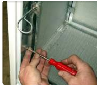
Pre & secondary filter holding frames
